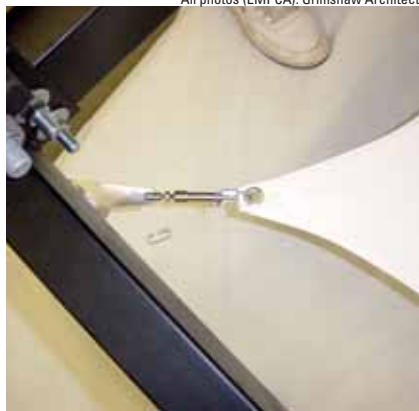
A detail of the framing and suspension system used, for both aesthetic and acoustic reasons.
